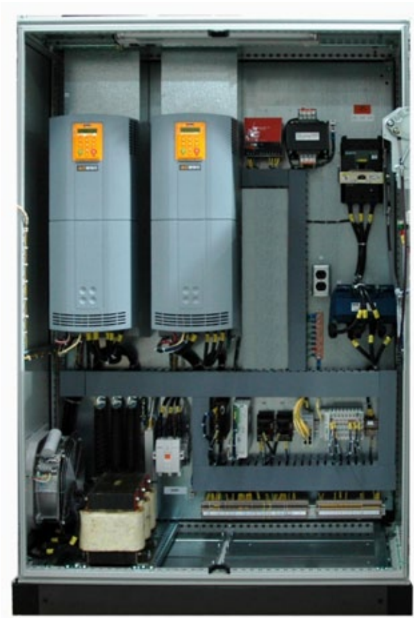
Illustration shows typical panel including AC690+ with AFE and additional system components.
