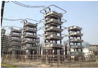
Series Capacitor Bank
