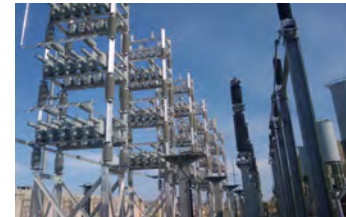
HV Shunt Bank
