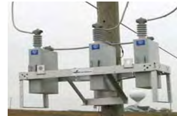
Pole-mounted Capacitor Bank
