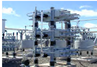
HV Filter Bank
