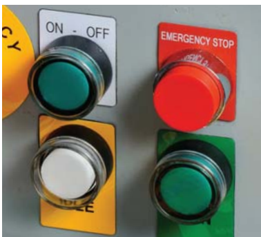
Control Panel Labels
