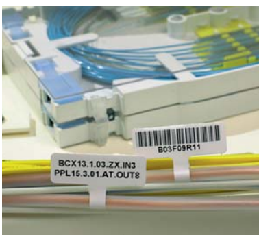
Fibre Optic Cable Markers
